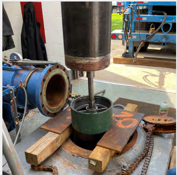
Pictured: New well pump being installed at Well 5. Photo courtesy of Kent Thompson
