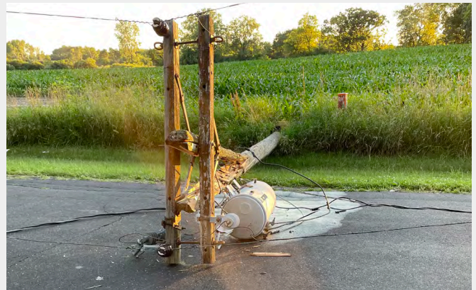
Pictured: A utility pole and transformer laying in the road after a tree fell on the power lines. Photo courtesy of Jill Weiss
