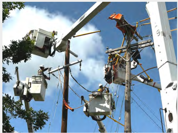
Pictured: Linemen relocating utility poles and electric lines in preparation for the Mandt Park project. Photo courtesy of Scott Adler
