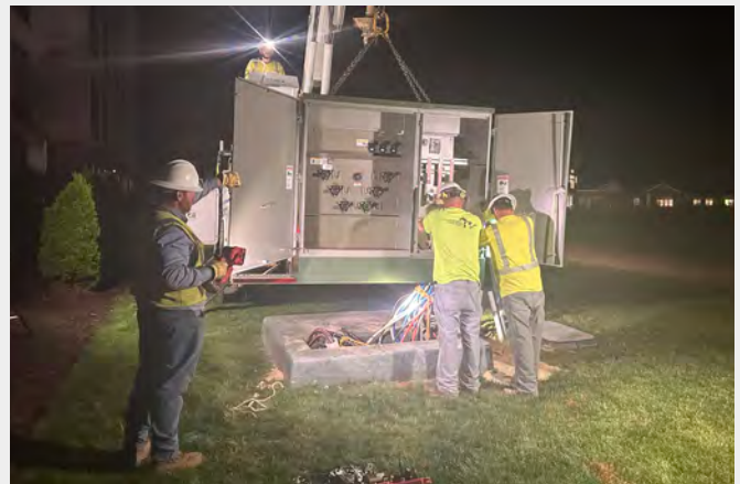
Pictured: Electric crew replacing the transformer at an area hotel after it was discovered to be leaking oil. Photo courtesy of Jill Weiss.
