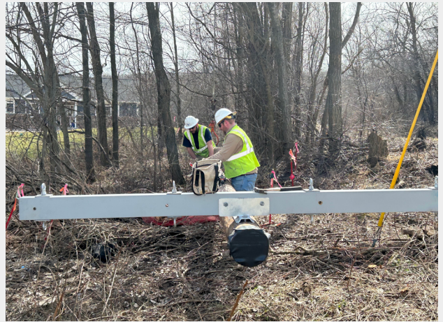
Pictured: Lineworkers Ryan J. and Andy R. replace utility poles on Halverson Road.
