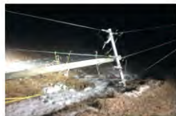
Caution Around Down Power Lines
